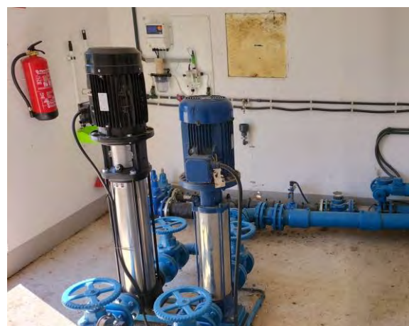
Figura 12. Interior caseta bombament Can Peirot.
